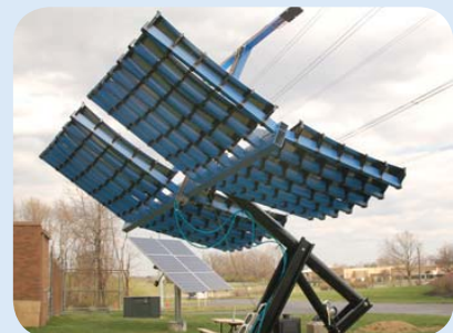
Solar power installations AEP is evaluating at its Dolan Technology Center.
